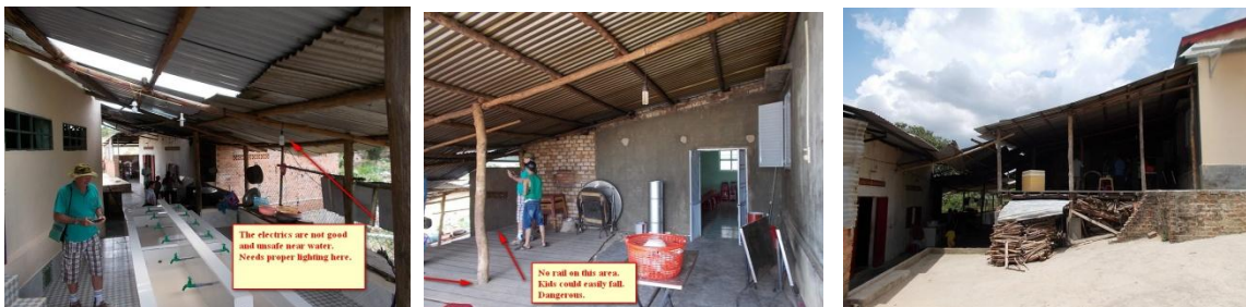
Vinh Son 4 Kitchen Area before (2015) but supposedly after construction!
